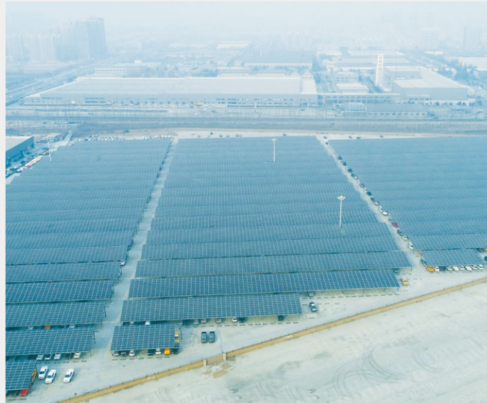
A Photovoltaic Project of ZNA's Zhongmou Plant
